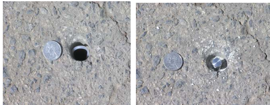
Photo 4 – Surface completions. Left: tubing coiled in hole. Removable plug installed to make flush with surface. Right: cemented flush to surface (hole slightly recessed purposely to enable fitting to be visible in photo).
