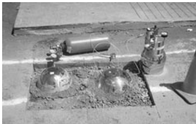
Surface-flux chambers installed on site.
